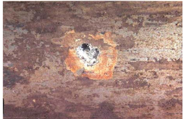
Figure 5 Pitting Due to Manganese Deposits (Photo Courtesy of Howell Image Sciences)
